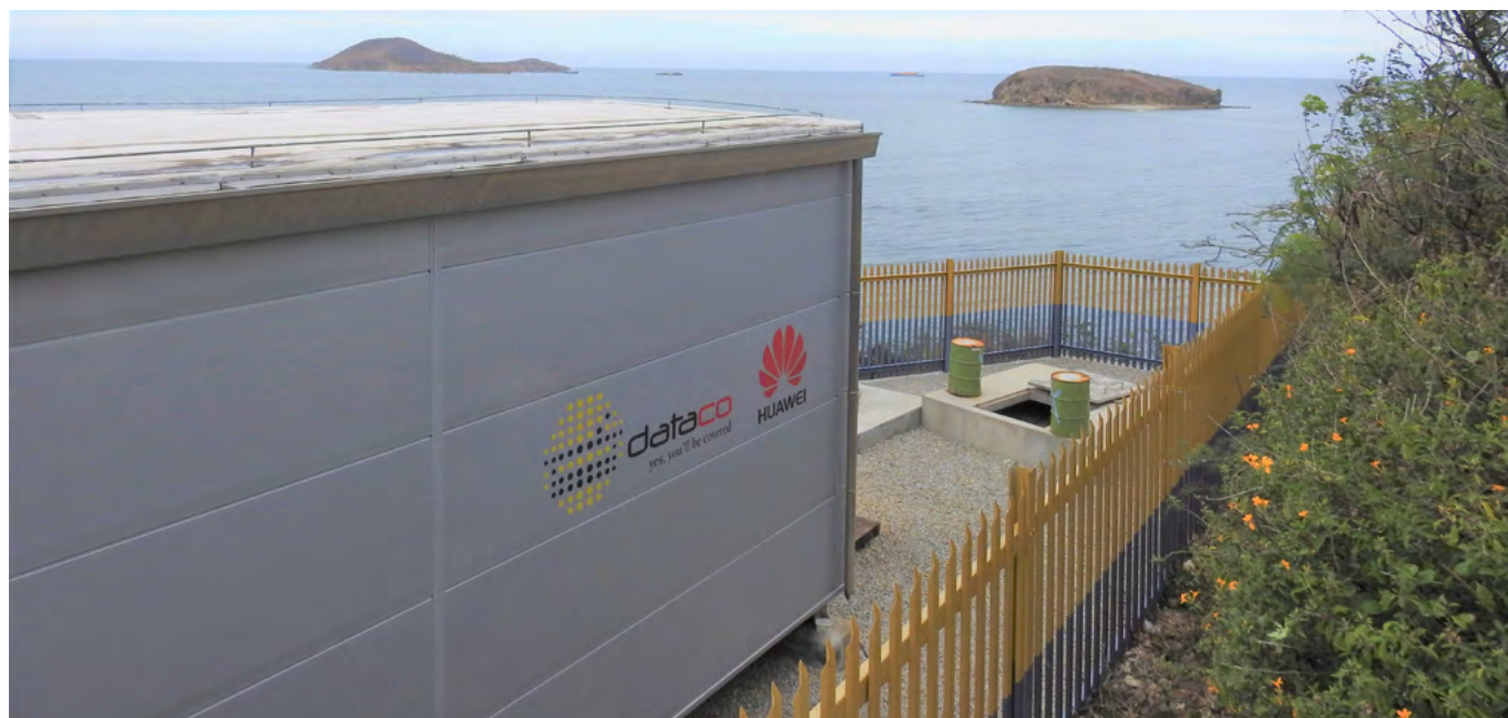
Figure 3. KSCN Landing Station
